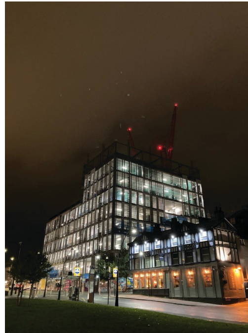
Sheffield Hallam University's new building under construction on the corner of Howard Street and Paternoster Row. (Photo © Owen Anthony)
