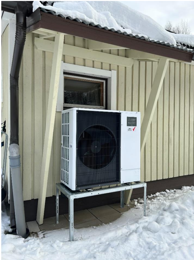
Source: Air Source Heat Pump (external unit), Finland. Copyright: Mari-Sohvi Miettinen
